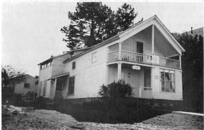
The Captain William Webster home, built by Lafayette Balch in 1854-55, is under renovation.
