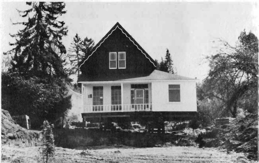
The Albert Balch house is ready to be moved forward during renovation.
